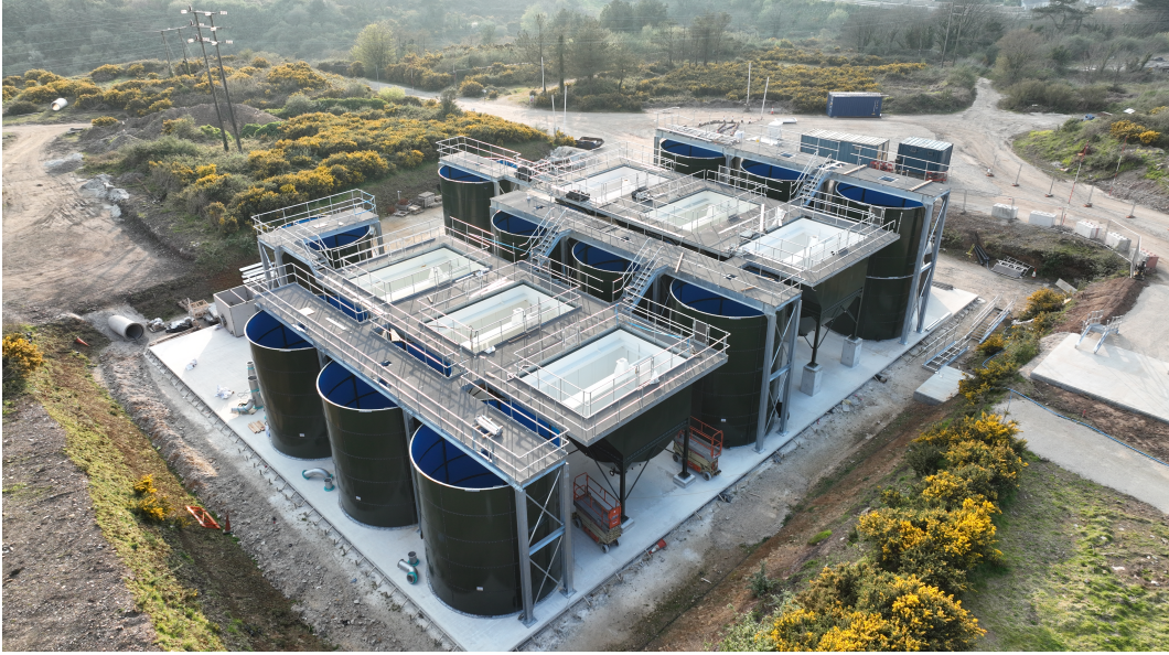
Aerial view looking northwest of the water treatment plant with walkways being assembled.
