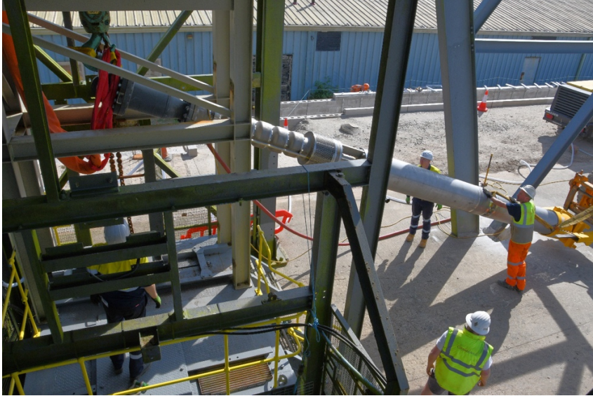
Photo 1. Hoisting the KSB submersible pump into vertical position under the NCK Headframe.
