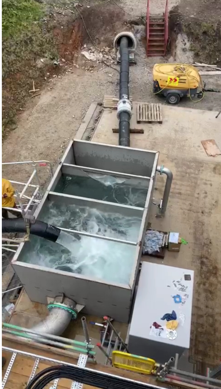
Photo 3 – Water being pumped through the water discharge tank and being re-circulated into the old mine workings during pump commissioning.
