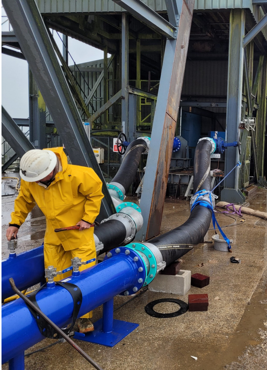
Photo 1 – Pre-commissioning of pipes leading from submersible pumps in NCK shaft to the Water Treatment Plant
